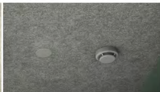
預留煙霧感應器和噴淋頭接入孔 Available for smoke sensors and sprinkler access holes
