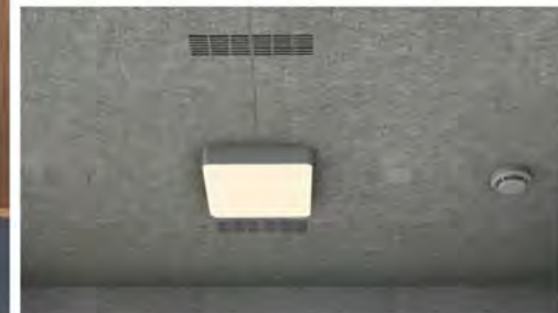
4000K自然光色溫 LED中央照明系統 4000K Natural Light Led central lighting system
